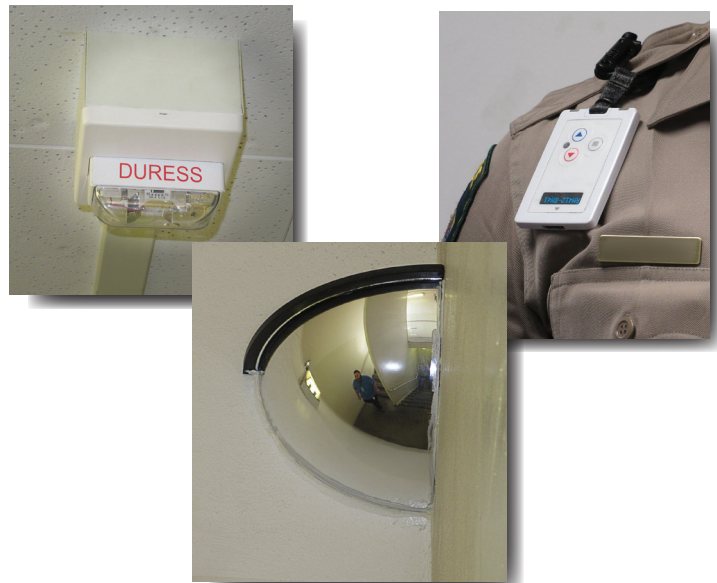
Examples of corrections (left to right): blinking alarm light, bubble mirror to see blind areas, personal alarm
