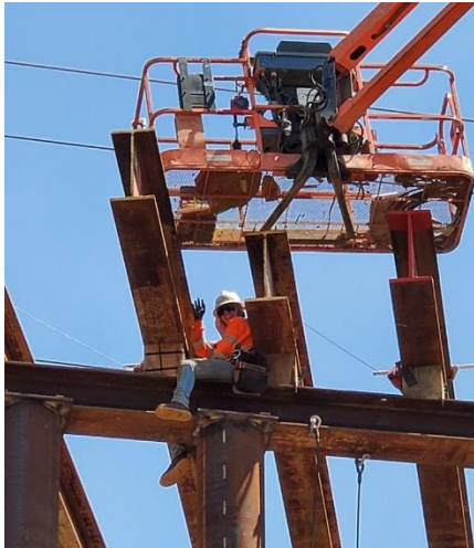
Chanel straddles a 100 foot high beam to secure wooden blocks to a stringer.
