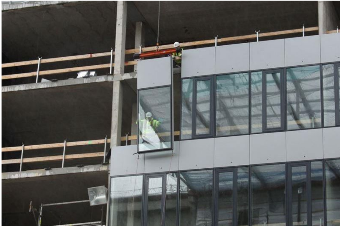
Figure 2. Installation of exterior building façade curtain wall. Curtain walls are non-structural building exterior coverings made from lightweight materials such as glass or aluminum. (Photo Credit: mornglass.com)
