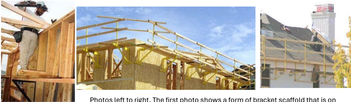
Photos left to right. The first photo shows a form of bracket scaffold that is on the interior of an exterior wall and does not meet Title 8 scaffold requirements. The next photo shows the current method under 1716.2 at the second story exterior. This is currently required in California. The last photo, once again shows a fully framed home.
